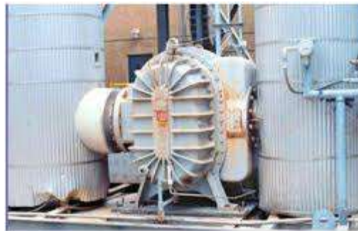
Figure 1 - Roots-type positive displacement blower at a petrochemical plant. (Source: Lubrication Systems Company, Houston, Texas)
